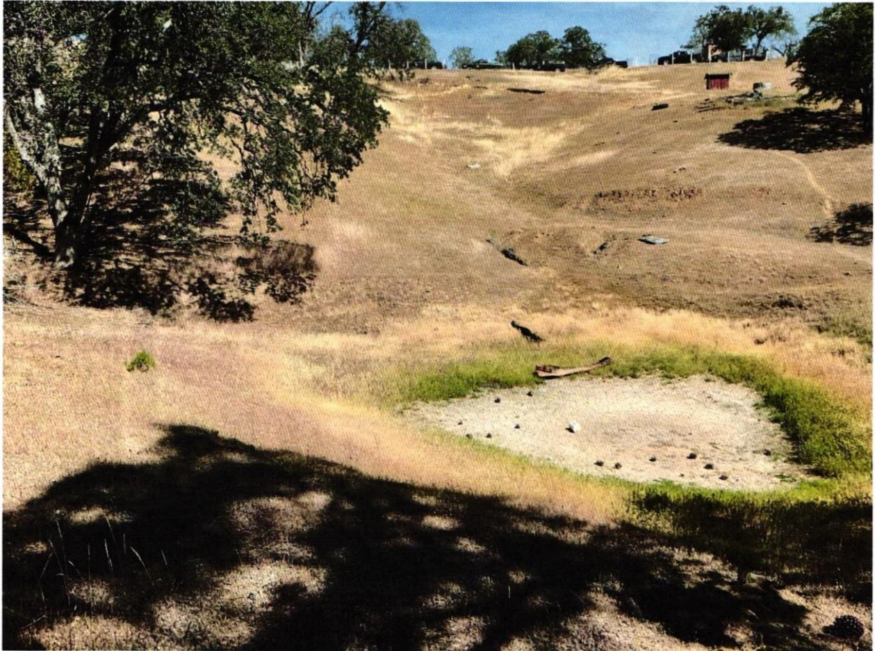
Photo #6, Site ID "PP-6". Placement of tire, metal siding, plastic buckets, other household trash and miscellaneous debris in stream channel and onstream reservoir.
