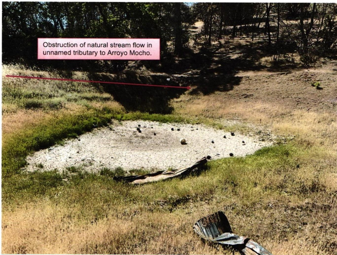
Photo #1, Site ID "HAPT-1". Construction of a dam, placement of fill, and obstruction of natural stream flow in an unnamed tributary to Arroyo Mocho. Creation of onstream reservoir due to obstruction of natural stream flow.
