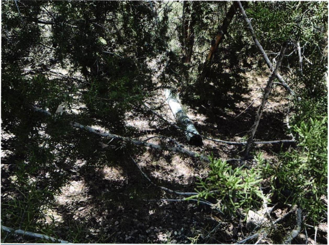
Photo #3, Site ID "MP-4". Five feet of broken off corrugated piping that is the result of a misaligned overflow pipe that was perched above the stream. Broken off piping deposited within 50 ft of waters of the state.
